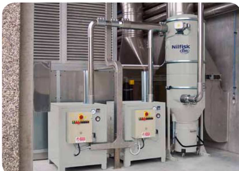
Centralized vacuum system in a chemical company: 2 vacuum units, 1 filter silo
